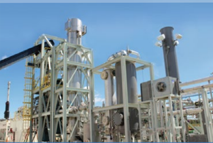
Sierra Energy Demo Plant at Fort Hunter Liggett, Monterey County
